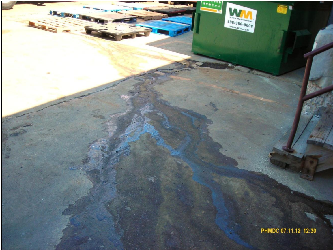
Photo 19: staining from chronic leaking of dumpster leachate.
