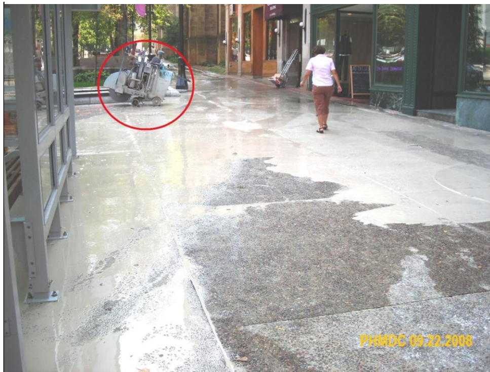
Photo 1: concrete slurry running down the sidewalk. The concrete saw is circled in red.
