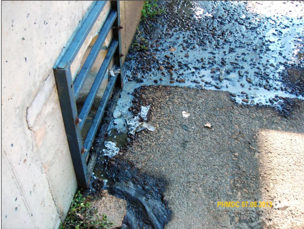
Photo 20: pooled leachate and severe concrete etching from chronic dumpster leak.
