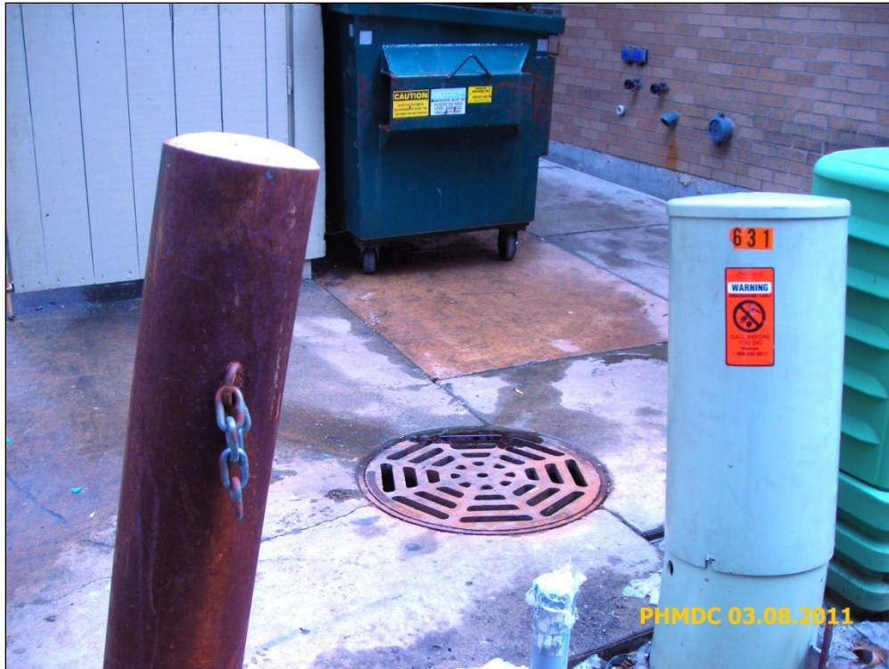
Photo 4: overfilled container leaking used cooking oil to storm sewer.
